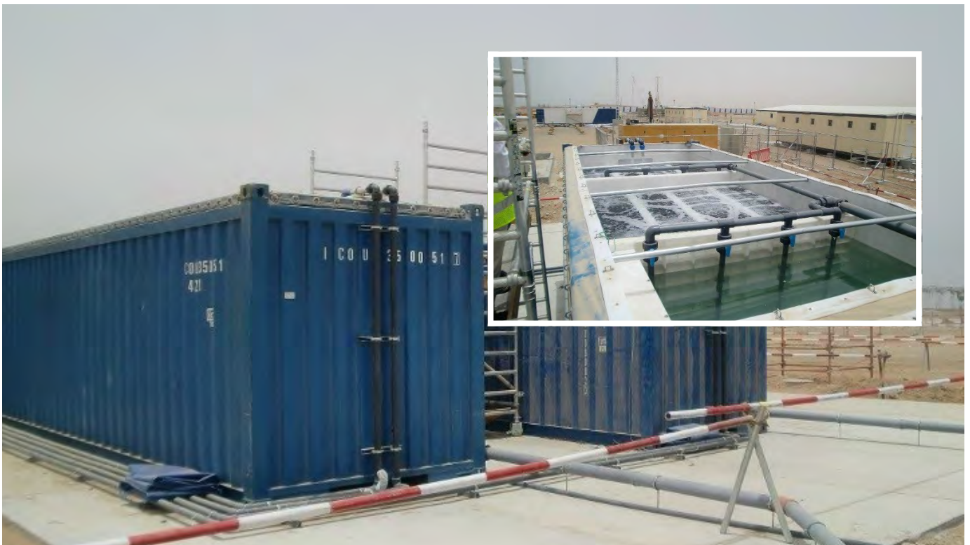
Labour Camp, Carillion Alawi LLC, in Oman. There are 2 x BioContainer BioMax 40' near a beach resort.
